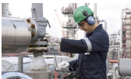
The Sniffers' leak detection tools
